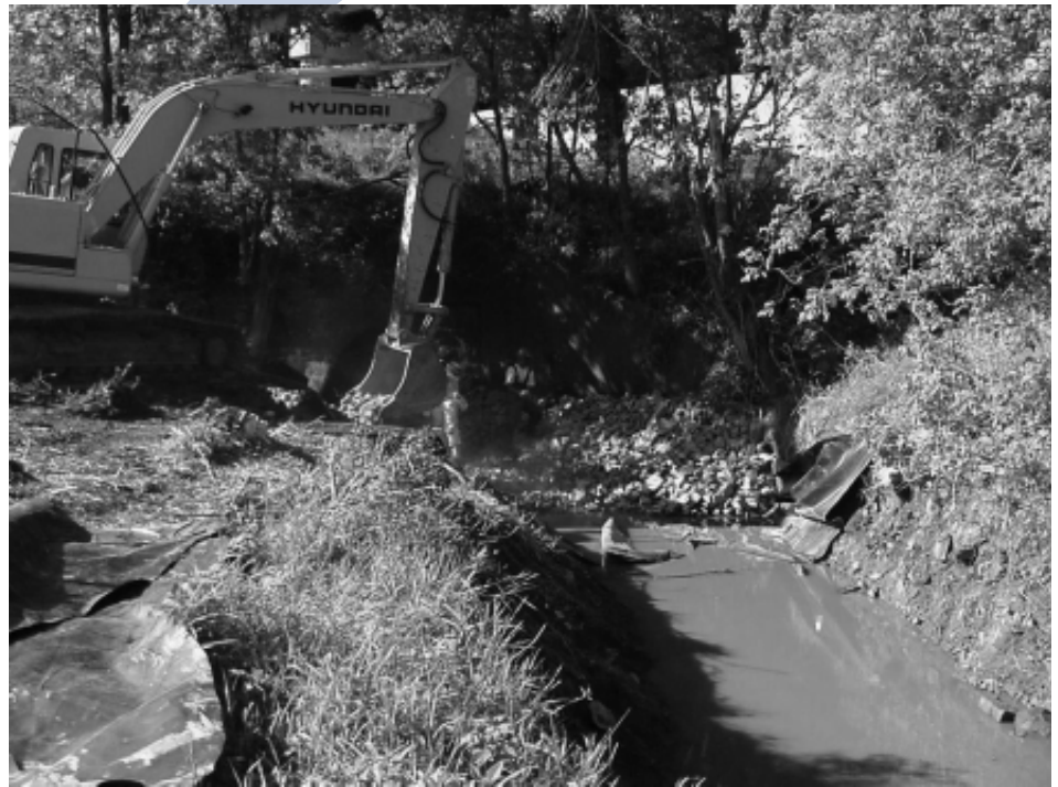
The natural water flow through Newton Creek in Superior, Wisconsin was diverted to remove contaminated sediment. Before the flow was restored, the creek was lined and covered with sand, gravel, and rocks to create a more natural shoreline and provide fish habitat. (Photo courtesy of U.S. EPA GLNPO)
